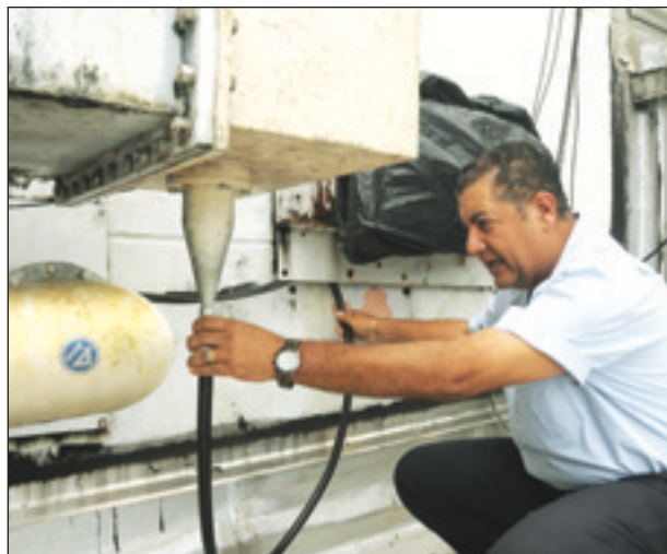
Angel, WP3R, connects LMR-900 feed line to a waveguide-to-coax transition, just outside the transmitter room.
